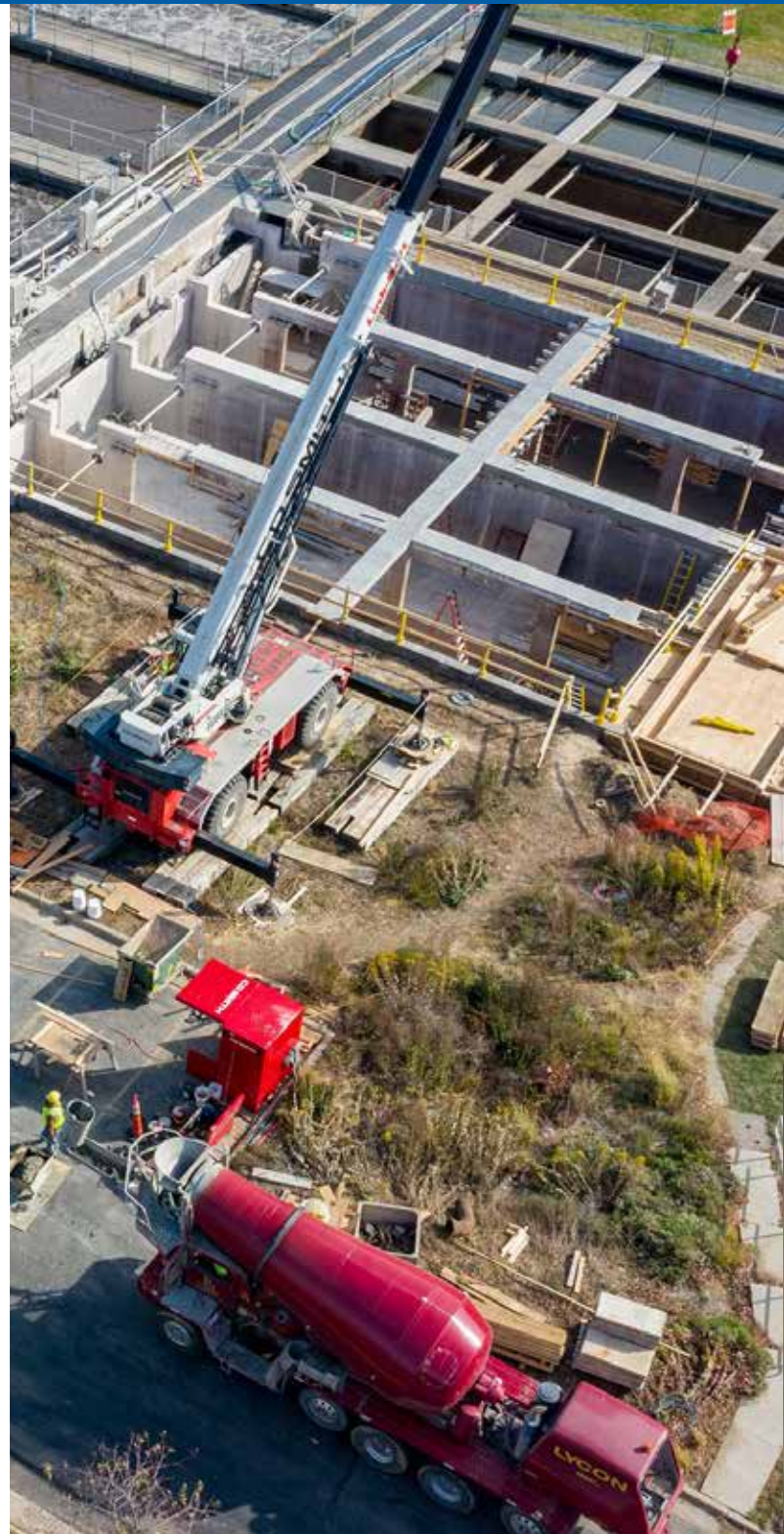
Large construction projects, whether on the Nine Springs Treatment Plant campus or offsite, require years of strategic planning before work can begin.
