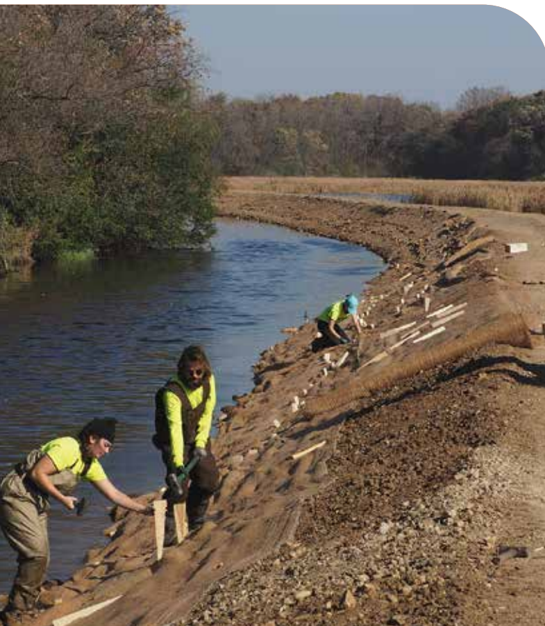
Contractors work to rebuild bank slopes and enhance habitat to stabilize the earthen dike at Grass Lake.
