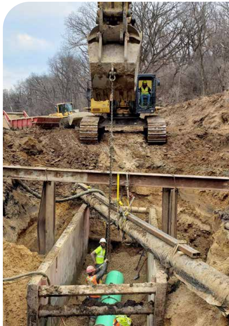
Crews work on installing the Pumping Station 17 relief force main in 2021. This pipeline will increase capacity for future development in the Lower Badger Mill Creek watershed.
