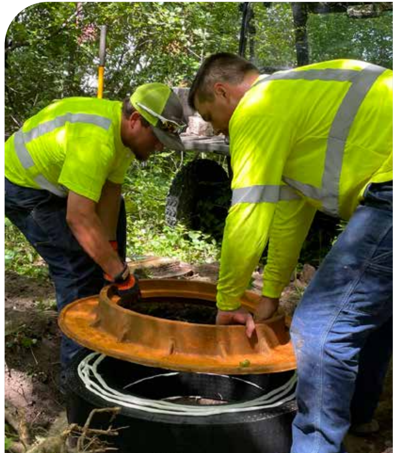
Collection System Services staff Ben Vehlow and Derek Steinhorst raise a manhole casting by using two rings, a non-rocking frame and a sealed cover to help reduce inflow and infiltration (I/I) in sewers.
