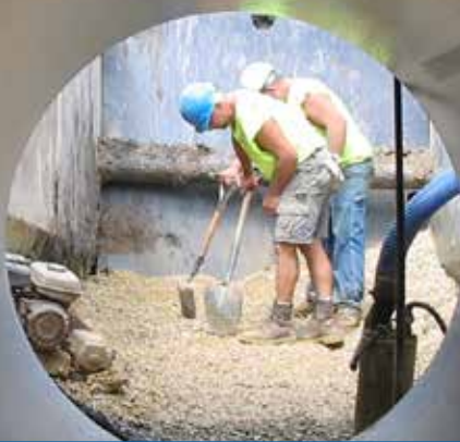
A look from inside the pipe as work is being done on a section of the Northeast Interceptor.
