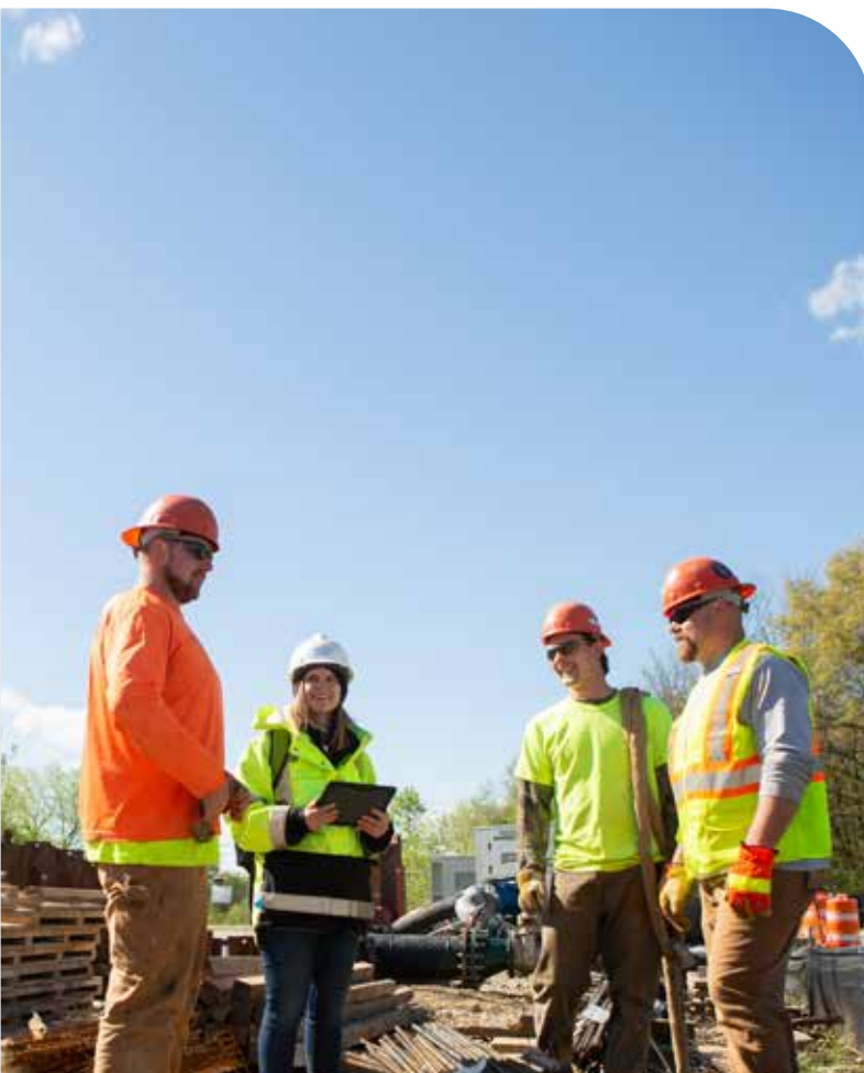
Project engineer Rachel Feil talks with contractors on the Nine Springs Valley Interceptor Capacity Improvements project site between McKee Road and Dunn’s Marsh.
