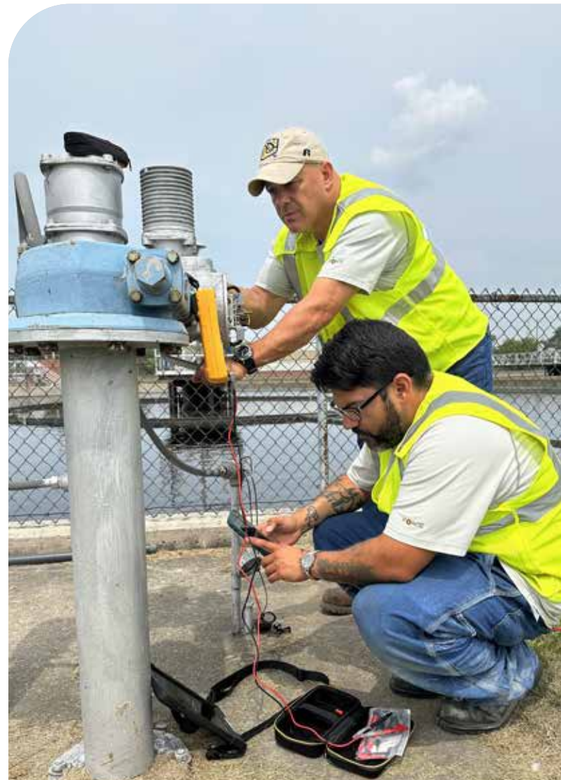
Electricians Roy Wells and Roy Rodriguez troubleshoot the actuator for a final clarifier at the Nine Springs Wastewater Treatment Plant.
