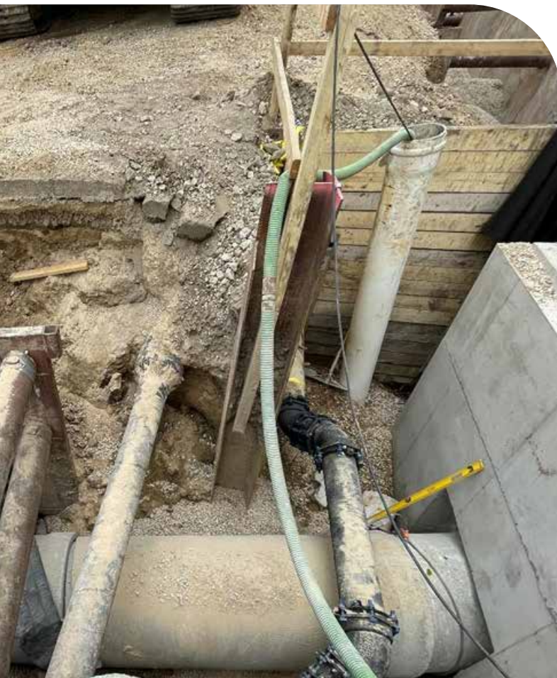
The 2023 repair of the West Interceptor at Marshall Park on Allen Boulevard required repairs to 60 feet of 30" pipe and three structures.
