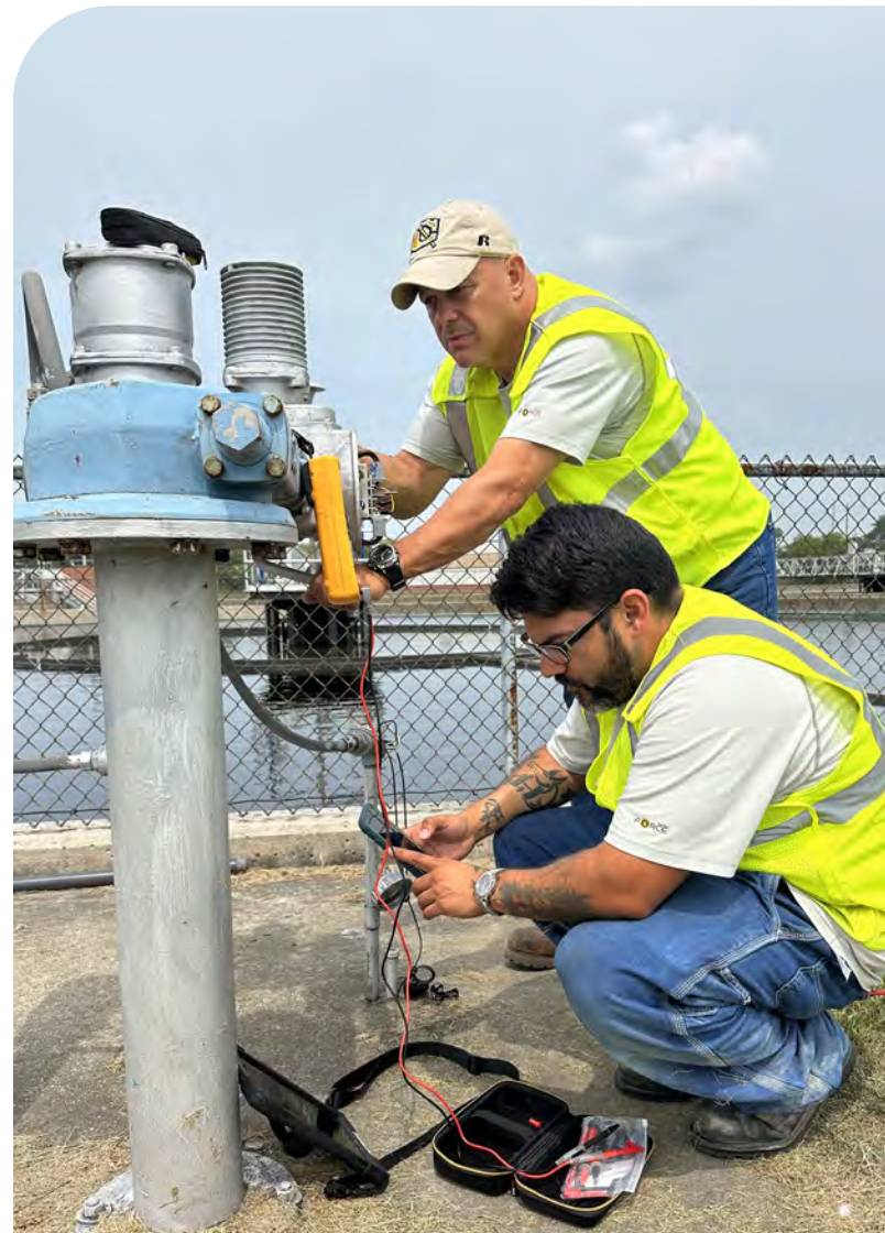
Electricians Roy Wells and Roy Rodriguez troubleshoot the actuator for a final clarifier at the Nine Springs Wastewater Treatment Plant.
